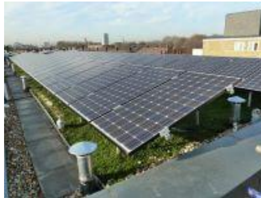
Figure 3.14: Green Roof Solar Panels
