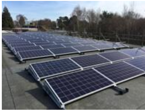
Figure 3.9: PV Mounts South Facing
