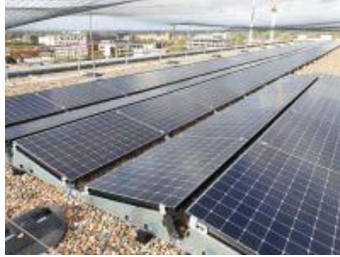
Figure 3.10: East/West Facing Solar Panels
