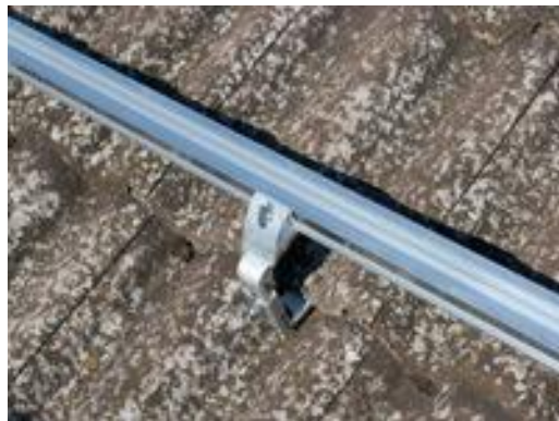
Figure 3.6: Roof Tilted Mount
