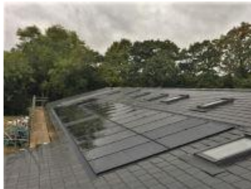
Figure 3.8: Solar Roof Panel with no Penetration of cement
