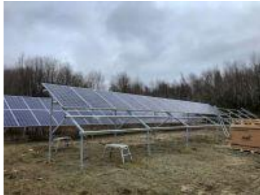
Figure 3.12: Ground Mounted Solar Panels
